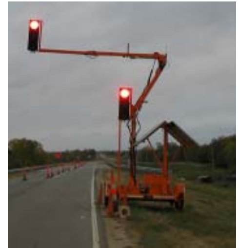
The traffic light that controls traffic over the partially closed bridge on K-4 has recently delayed traffic between Highway 81 and school. The scheduled completion date for the bridge repair is Oct. 28. (Photo by Krisanna Graham)
