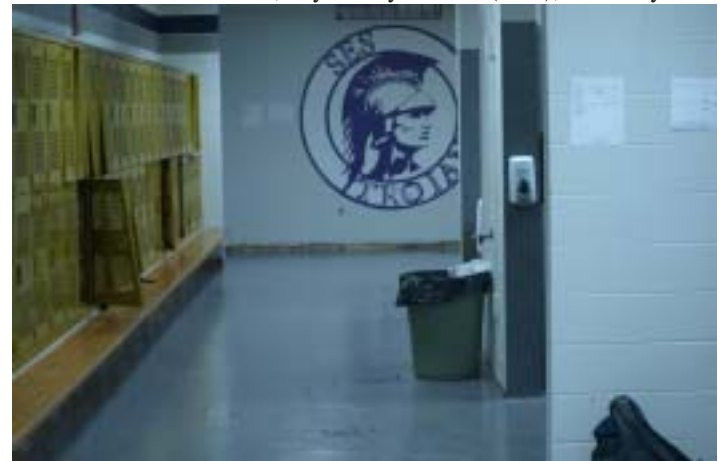
The boys' locker room got a new surface after the old carpet was pulled out at the end of the 2008 school year. The locker room is where senior Zach Downey fell. His fall required him to get seven staples. (Photo by Max McClure)
