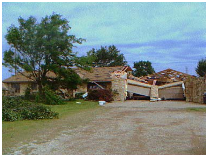
The Hettenbach's house (pictured) suffered enough damage from the June 11 tornado that it had to be torn down. Construction on their new house is hoped to be completed by March. (Photo courtesy of Sara Hettenbach)
