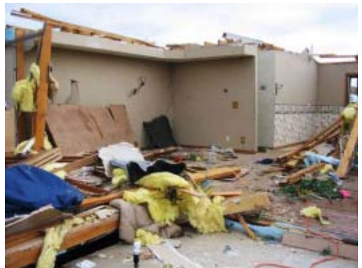
The Losey's house (pictured) suffered extensive damage after the tornado. They lost their entire upstairs and roof in the natural disaster. (Photo courtesy of Losey family)
